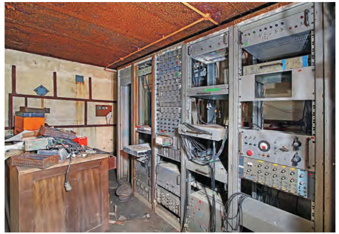
Although the P1 firing bay has been backfilled the semi-underground control room is still accessible with much of its control and recording equipment still in situ accommodate complete missiles which were lifted onto the stand by crane.
